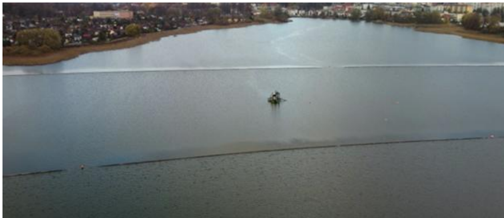
Figure b.29. Sediment removal from the part of Karczemne Lake – geomembrane curtains were used for separation of regulation area from the rest of lake (source: Kartuzy WWTP)
