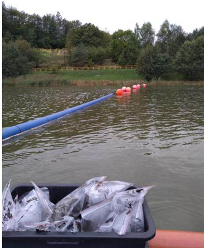
Figure b.27. Pipeline for sediment hydrotransport to Kartuzy WWTP (photo: J. Grochowska)
